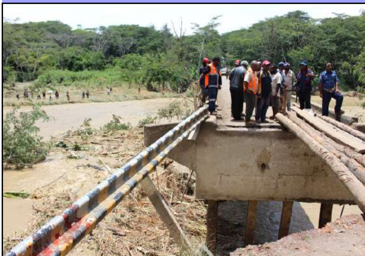
Recently destructed Bena bridge in Eastern Highlands Province due to heavy rains which affected the movement of coffee to Lae, Morobe Province
