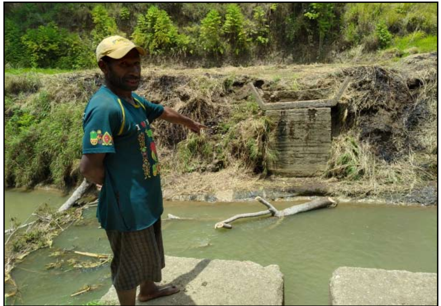
A local in Magitu pointing to the damaged bridge.
