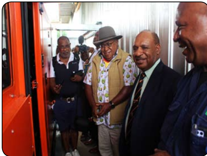
Coffee Minister Hon. William Bando turning on the main switch for the 200 KVA genset at the Anego Coffee factory during the reopening of the factory on Friday, February 14th, 2025.
